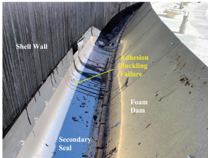
Figure 8. Buckling of metallic secondary seal compression plate due to polymer extrusion adhesion to shell wall.
